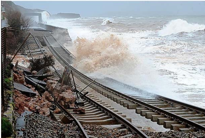
Figure 16. The main railway line to Cornwall and Devon was demolished at Dawlish by storms, which hit the UK in February 2014 (Courtesy: Network Rail).
