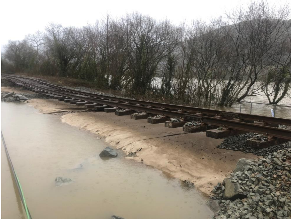
Figure 4. Washouts in 2020 leading to suspended track on the Conwy Valley Line (source: Network Rail)
