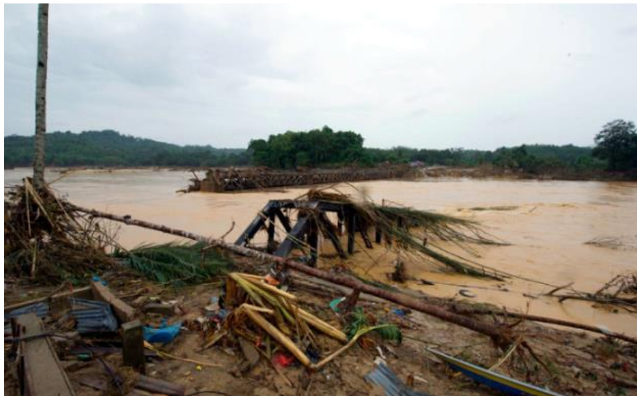
161 162 Fig. 3. Washaway of railway tracks occurred in Malaysia East Coast Line railway 163 bridge, which cross Nenggiri River in Kemubu, Kelantan had totally lost due to mas- 164 sive flood in December 2014. (Courtesy: Malaysian Department of Public Works)
